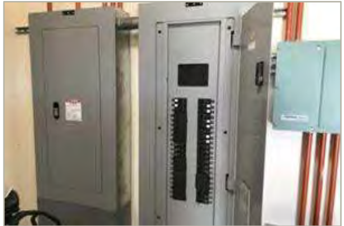
10 - MAIN ELECTRICAL PANEL
