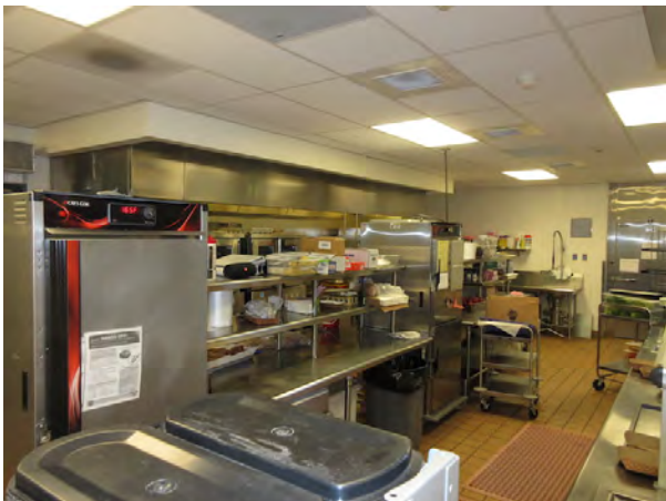
North Terrace K-8 School Kitchen
