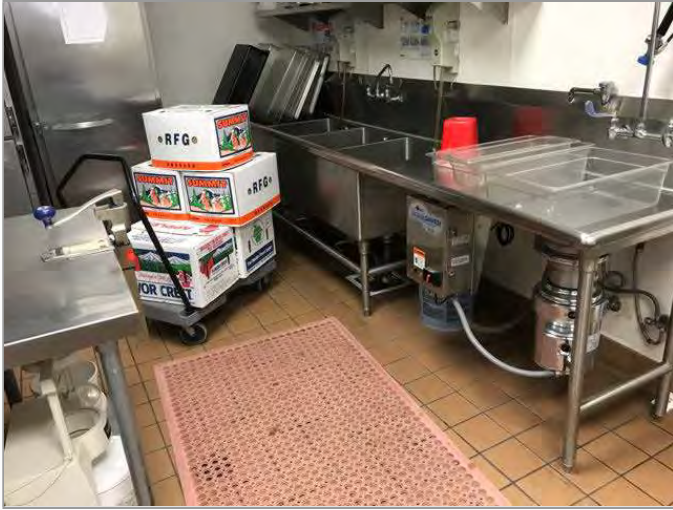
Kitchen cabinets/sink clearance
