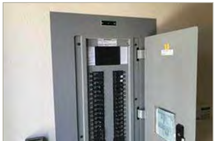
6 – MAIN ELECTRICAL PANEL
