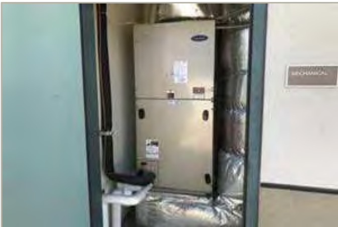
5 - INTERIOR FAN COIL UNIT
