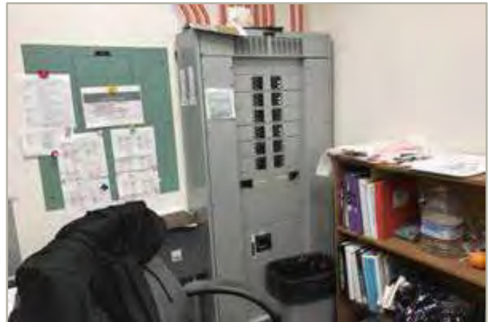
12 - MAIN ELECTRICAL PANEL
