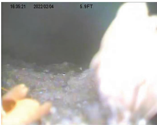
Sediment Build up in Pipe at 5.90 ft.
