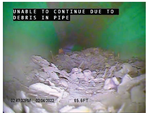
End of Run Due to Debris Blockage at 65.60 ft.
