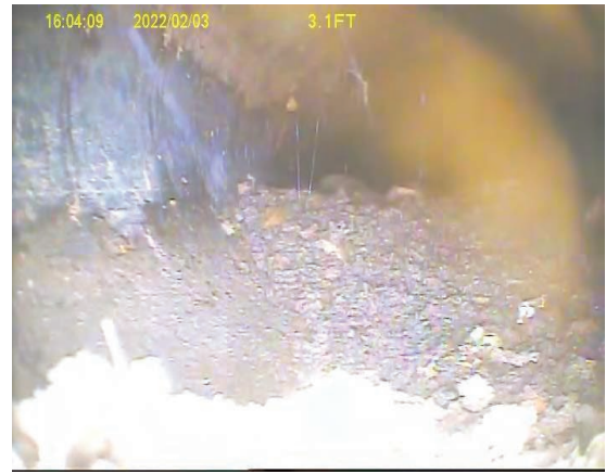
Sediment/Debris Build in Pipe at 3.10 ft.
