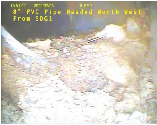
CCTV Starting Point
