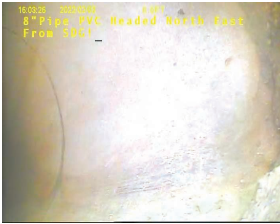
CCTV Starting Point
