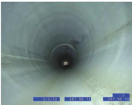
Typical Line Condition at 167.96 ft.
