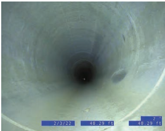
Typical Line Condition at 48.29 ft.
