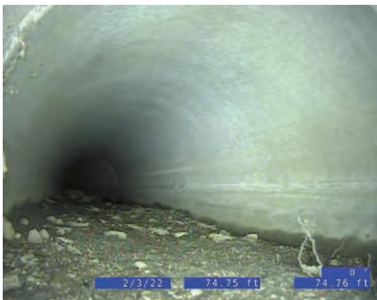
Line Runs to the Left at 74.75 ft.
