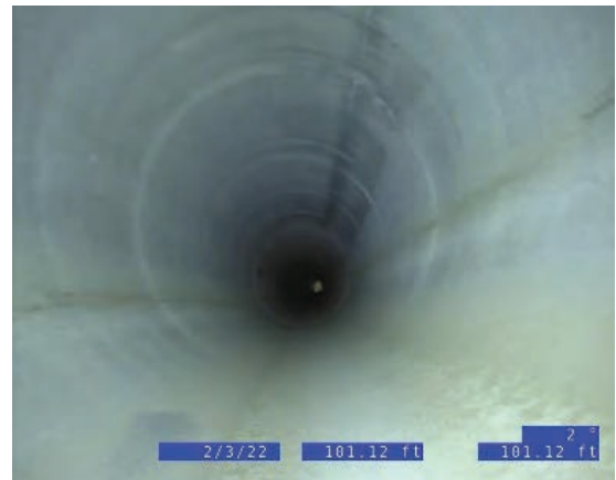
Typical Line Condition at 101.12 ft.
