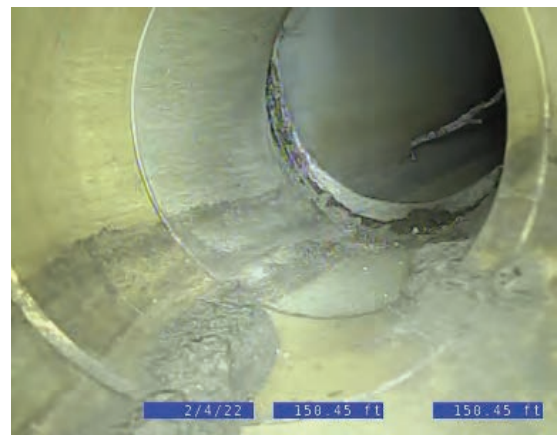
Line Runs to the Right/Offset in Pipe at 150.45 ft.
