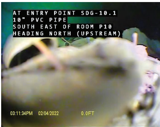
Debris Build up in Pipe at Starting Point
