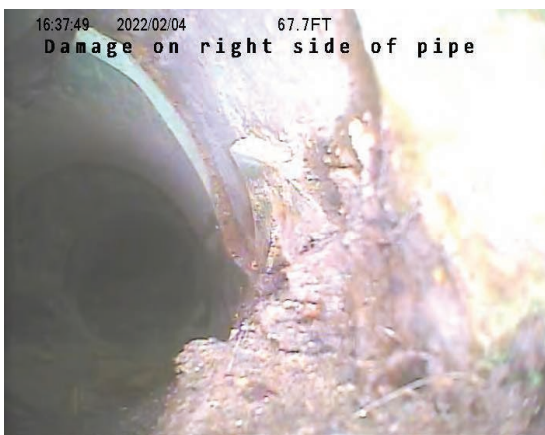
Damage on the Right in Pipe at 67.70 ft.
