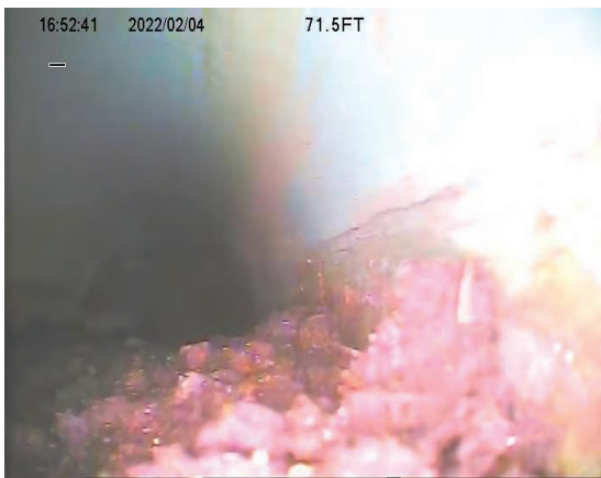
Sediment Build up in Pipe at 71.50 ft.
