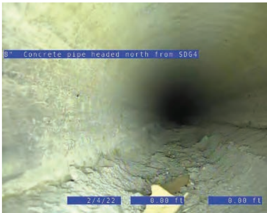
Sediment Build up in Pipe at Starting Point
