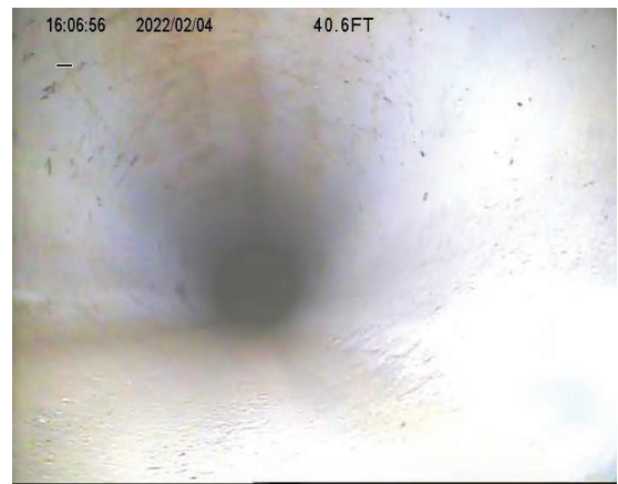
Typical Line Condition at 40.60 ft.
