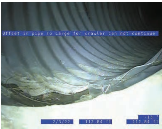
End of Run Due to Offset in Pipe at 112.84 ft.
