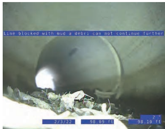
End of Run Due to Blockage at 98.09 ft.
