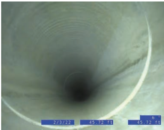
Typical Line Condition at 45.72 ft.
