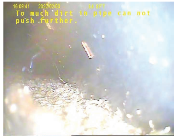
End of Run Due to Loss of Tension at 54.80 ft.
