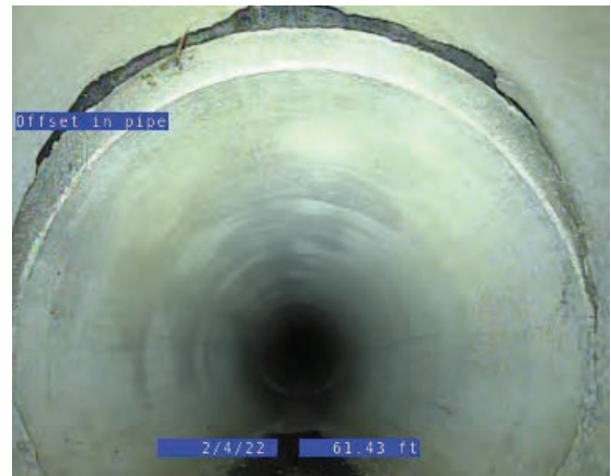
Offset in Pipe at 61.43 ft.
