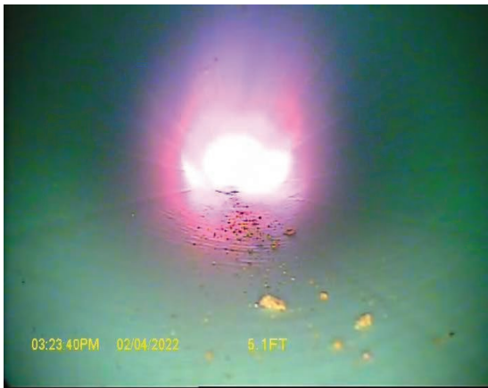
Typical Line Condition at 5.10 ft.
