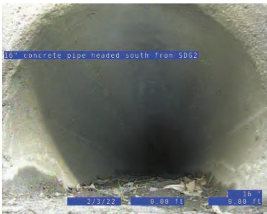
Sediment Build up in Line at Starting Point
