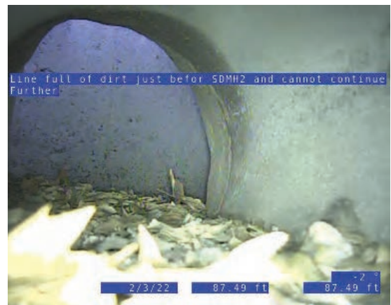
End of Run Due to Debris Build up at 87.49 ft.
