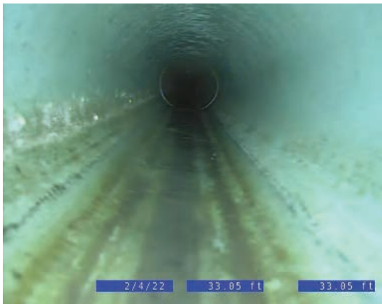
Typical Line Condition at 33.05 ft.
