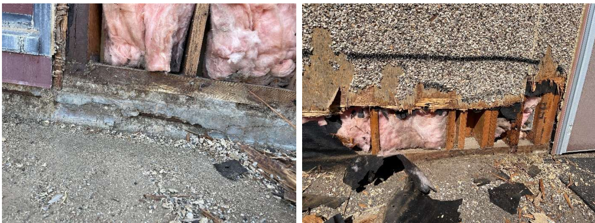
Building A & B Exterior Damage –
