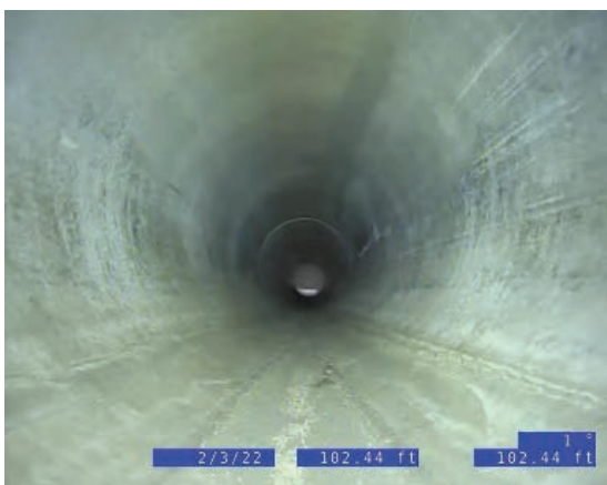
Typical Line Condition at 102.44 ft.
