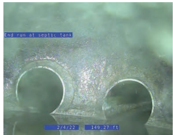
Ties Into Septic Tank End of Run at 149.27 ft.
