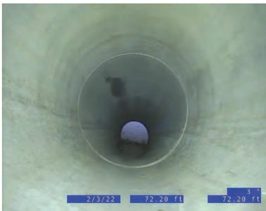
Typical Line Condition at 72.20 ft.
