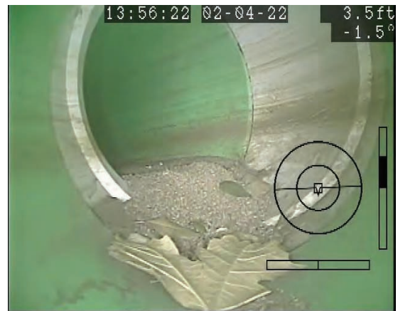
Line Runs to the Left at 3.50 ft.
