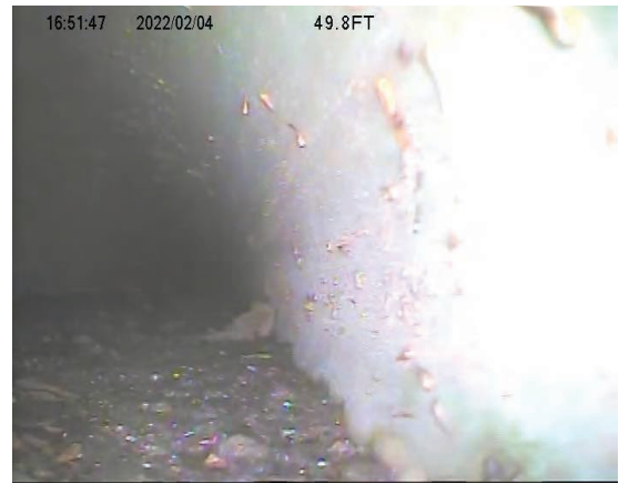
Sediment Build up in Pipe at 49.80 ft.
