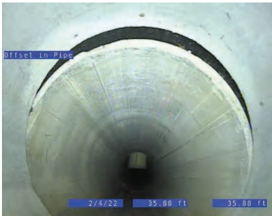
Offset in Pipe at 35.88 ft.
