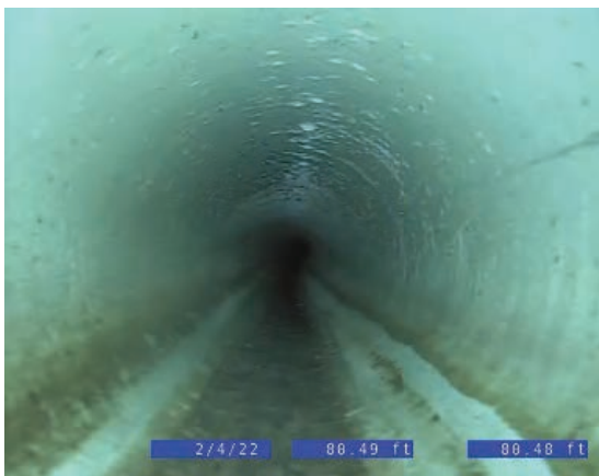
Typical Line Condition at 80.49 ft.
