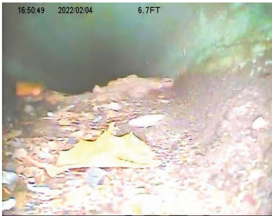
Sediment Build up in Pipe at 6.70 ft.
