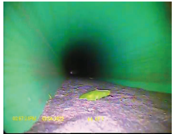
Sediment Build Up in Pipe Continues at 44.40 ft.
