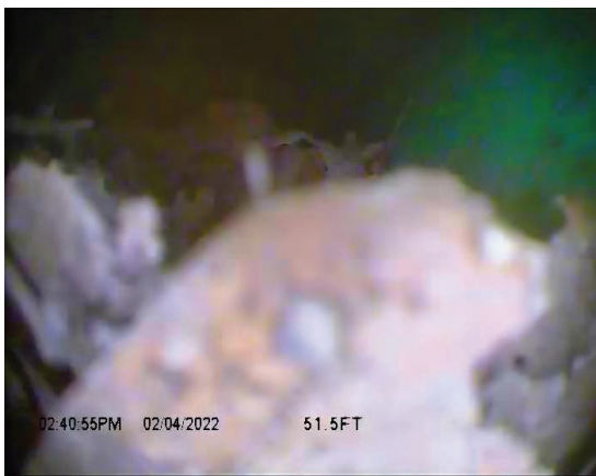
Debris Build up in Pipe at 51.50 ft.
