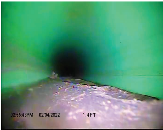
Sediment Build up in Pipe at Starting Point
