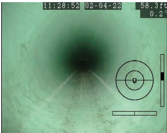
Typical Line Condition at 58.30 ft.
