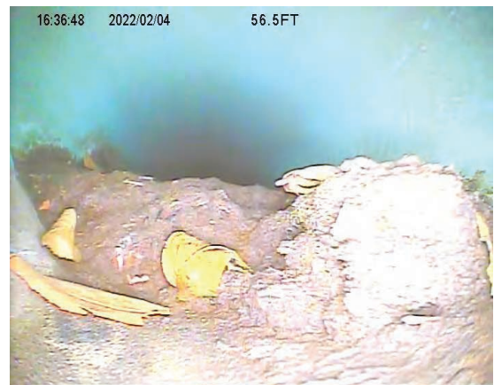
Sediment Build up in Pipe at 56.50 ft.
