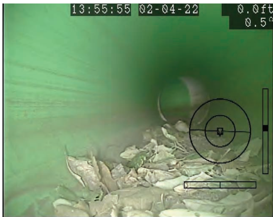
Sediment/Debris Build up at Starting Point
