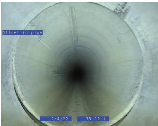
Offset in Pipe at 75.12 ft.
