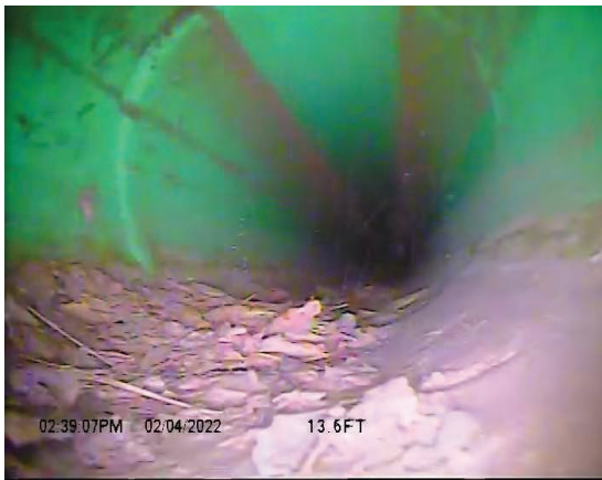
Debris Build up in Pipe at 13.60 ft.
