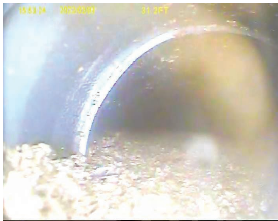
Sediment/Debris Build up Continue in Pipe at 31.20 ft.
