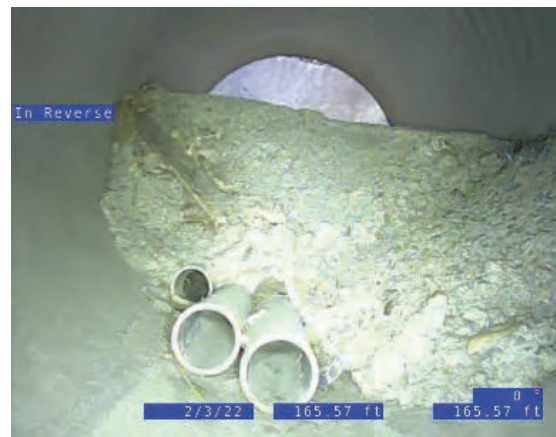
End of Run Due to Blockage at 165.57 ft.
