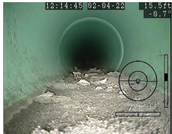
Sediment Build up in Pipe at 15.50 ft.
