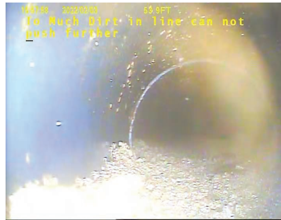
End of Run Due to Loss Tension at 53.90 ft.
