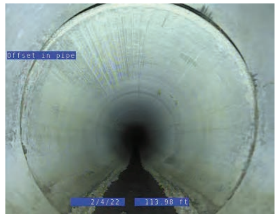
Offset in Pipe at 113.98 ft.
