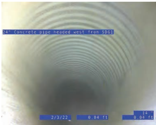
CCTV Starting Point
