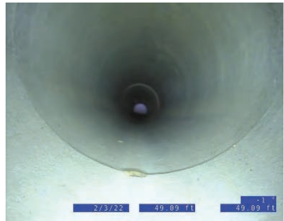
Typical Line Condition at 49.09 ft.
