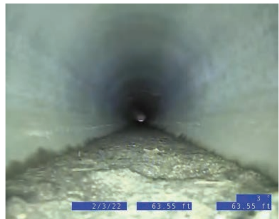
Sediment Build up Continues in Pipe at 63.55 ft.
