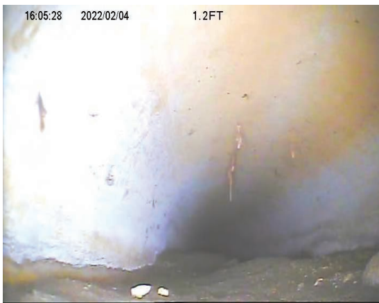
Sediment Build up at Starting Point
