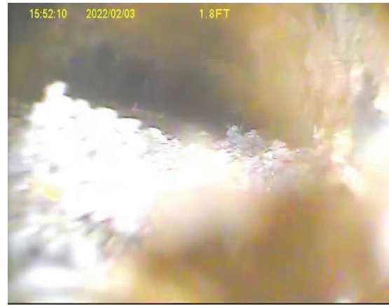
Sediment/Debris Build up in Pipe at 1.80 ft.
