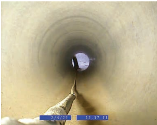
Typical Line Condition at 12.17 ft.
