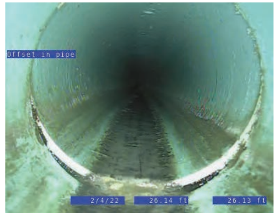
Offset in Pipe at 26.24 ft.
