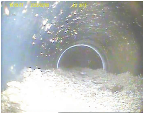
Sediment/Debris Build up Continues in Pipe at 42.30 ft.
