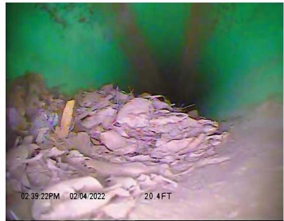
Debris Build up in Pipe at 20.40 ft.
