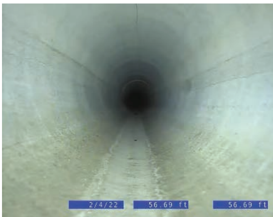
Typical Line Condition at 56.69 ft.
