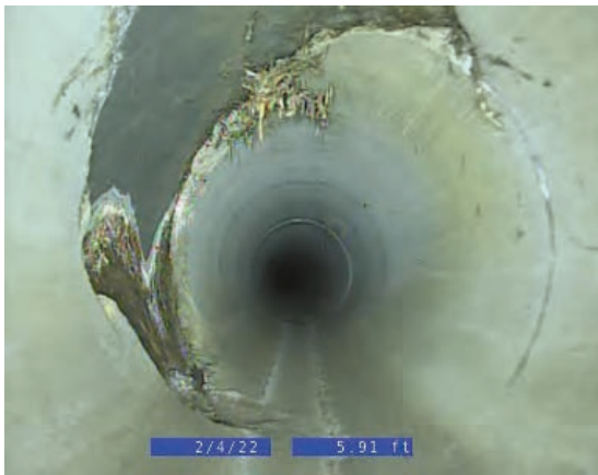
Damage on the Left at 5.91 ft.
