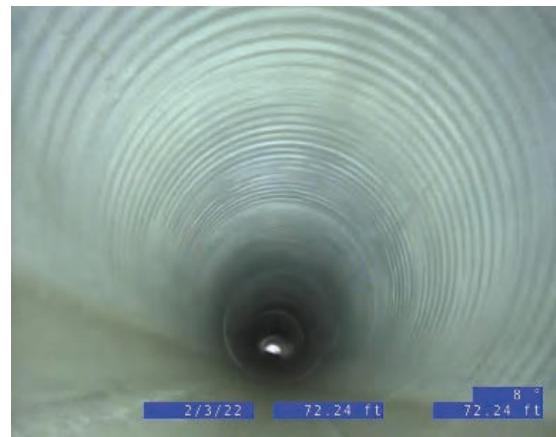
Typical Line Condition at 72.24 ft.
