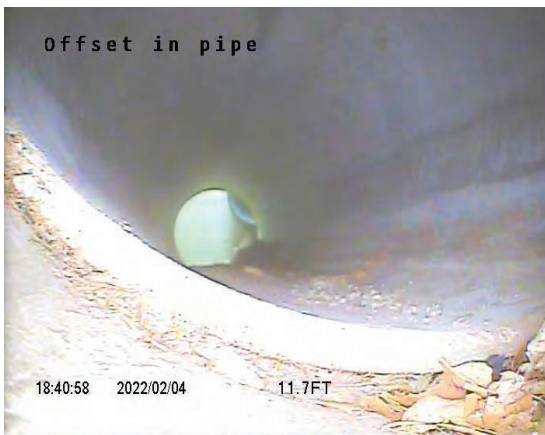
Offset in Pipe at 11.70 ft.
