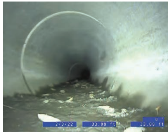
Sediment Build up Continues in pipe at 33.08 ft.
