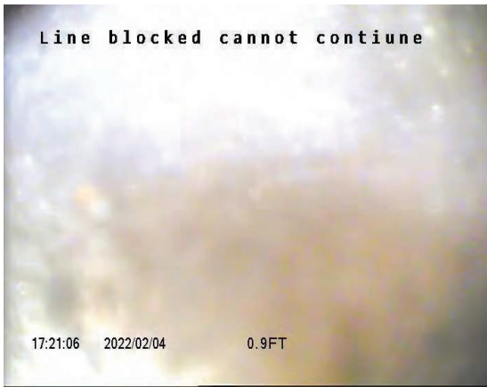
Line Blocked at Strating Point
