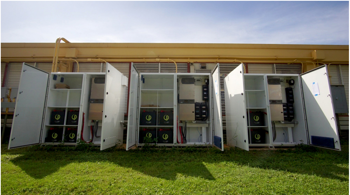
Simpliphi Hawaii Batteries
